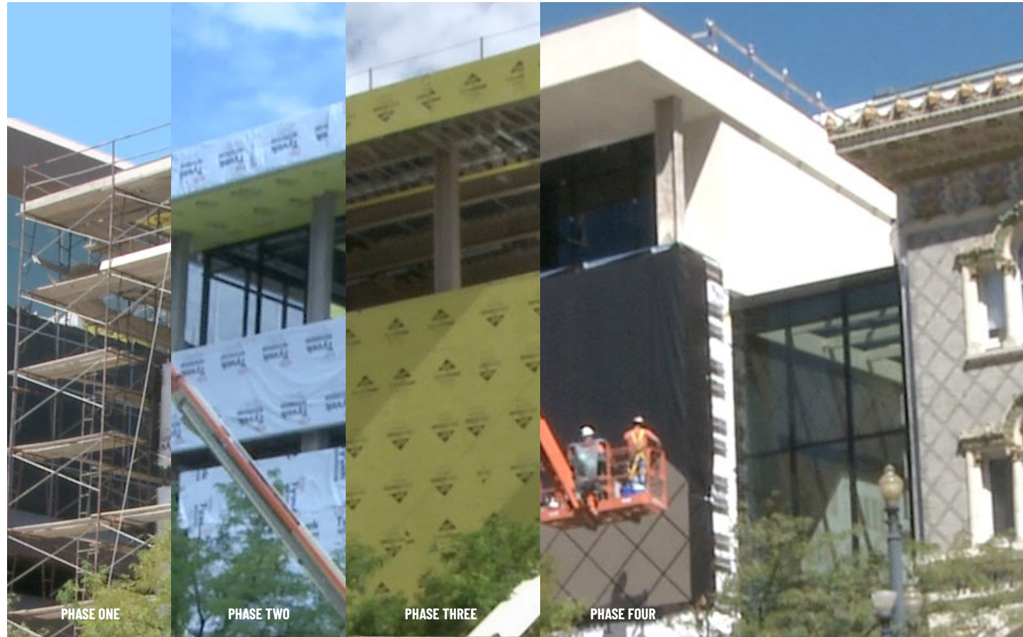
FREDERICK QUINNEY LAWSON BALLET CENTRE DURING CONSTRUCTION | PHOTOS PROVIDED BY BALLET WEST
